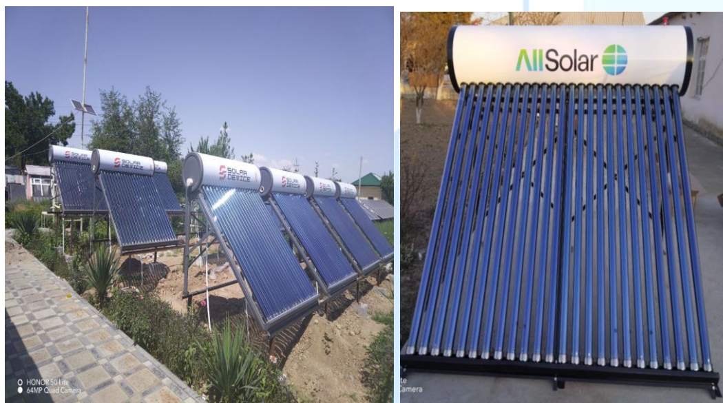
Figure 1 Solar Water Heating Collectors with Vacuum Tube
